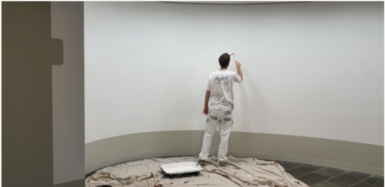
Once the new walls and spaces were built, the walls were repainted and time was allowed for off-gassing – the dispersal of any fumes or emissions from the paint
